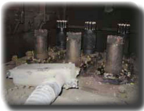
Photo 2: Electrical arc flash incident on 11 kV system.
